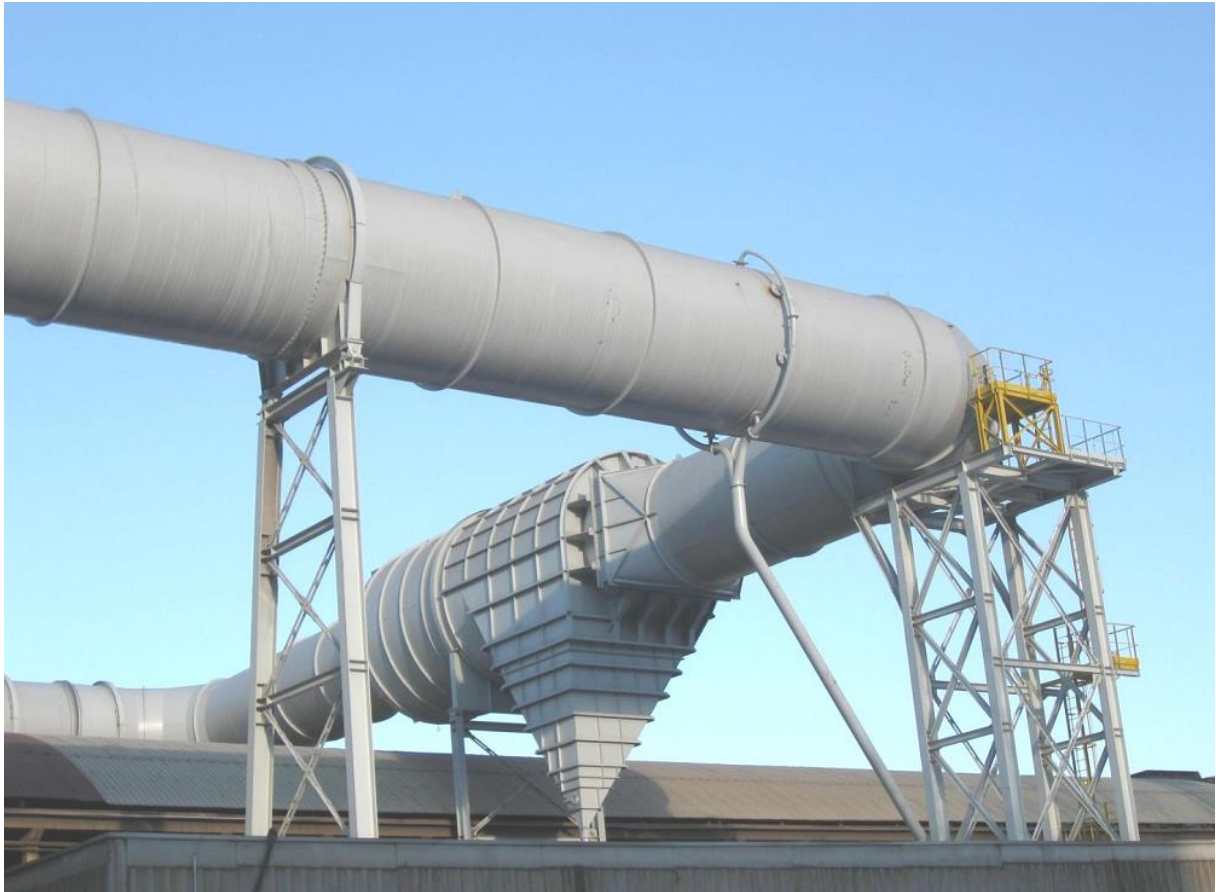
Fume suction and filtering system realized in 2010
